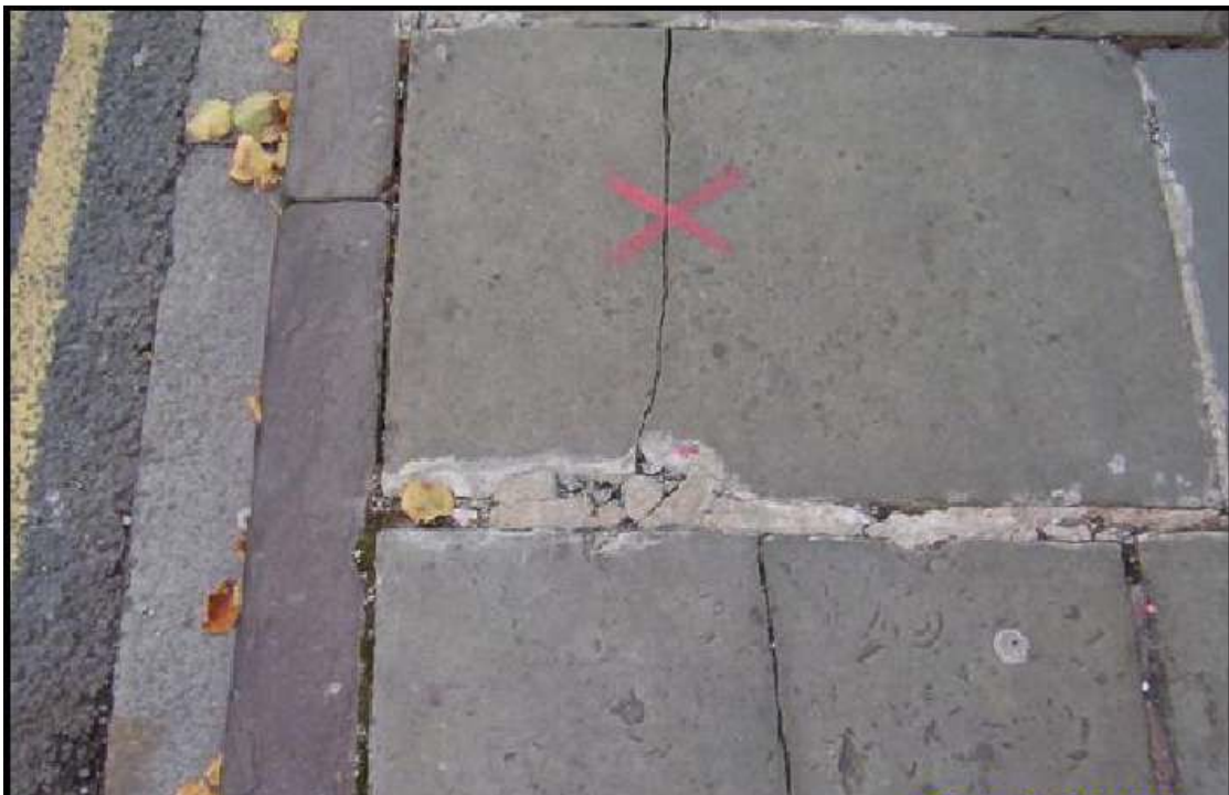
Footway, broken slabs, Link Footway: Target Response Time Cat 3.
