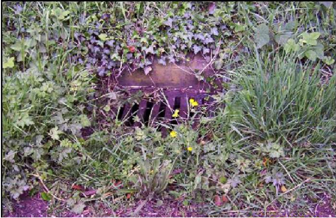
Blocked gully, Local rural: Target Response Time Cat 2.
