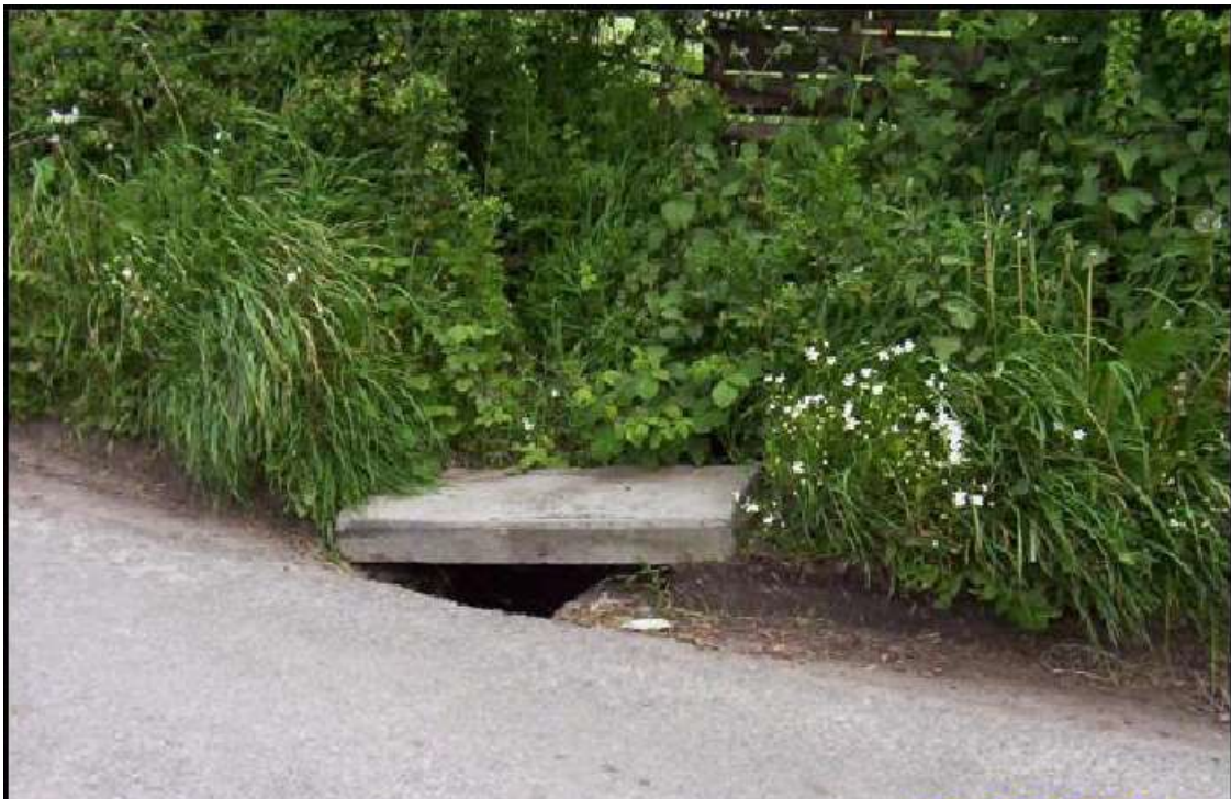
Damaged drain inlet: Target Response Time Cat 1.
