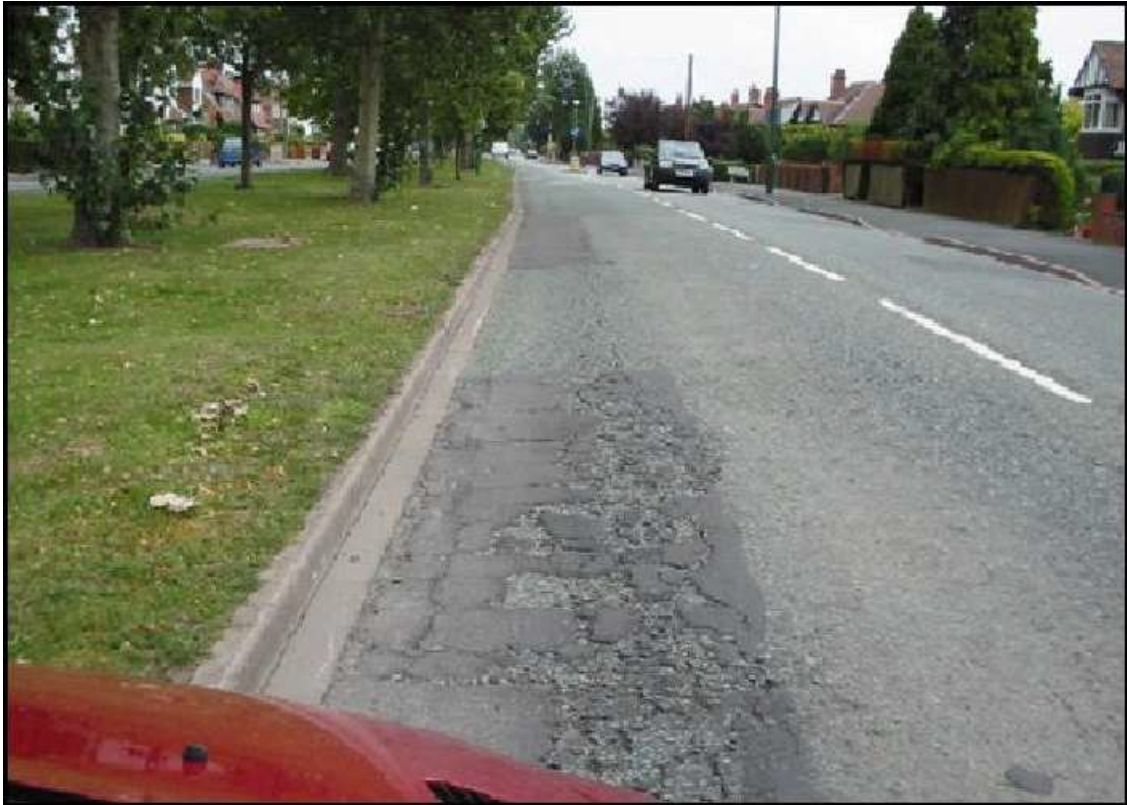
Fretting/Cracking Main Distributor urban, Type 3: Target Response Time Cat 1.
