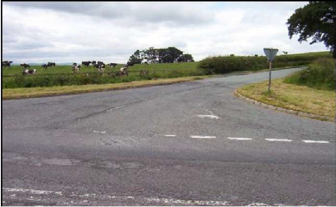
Faded road markings: Target Response Time Cat 2
