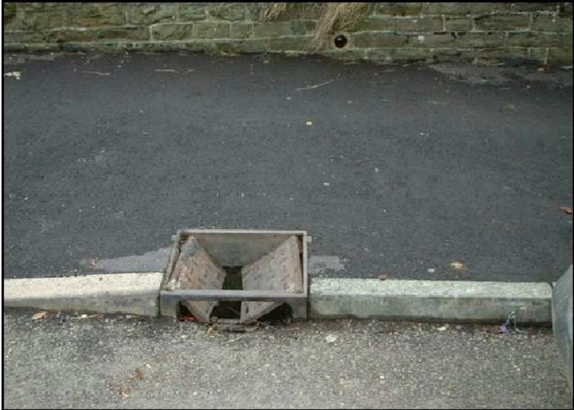
Broken cover, Secondary Footway: Target Response Time Cat E.
