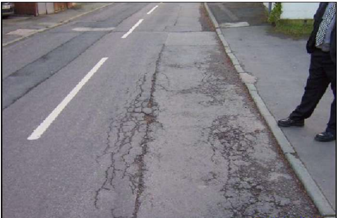
Secondary Distributor, surface crazing include in renewal programme.
