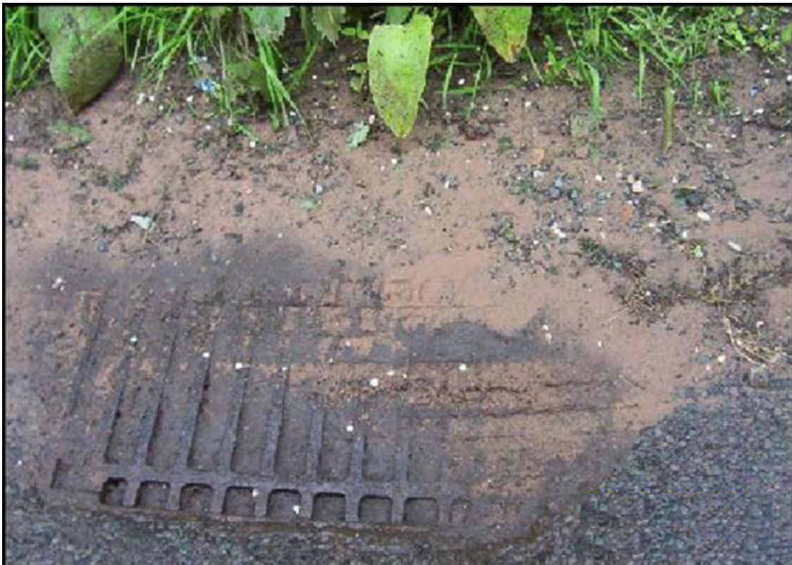
Blocked gully Secondary Distributor: Target Response Time Cat 1.
