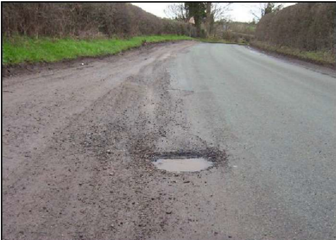
Pothole, Type 2 Defect on Secondary Distributor. Target Response Time Cat 1.
