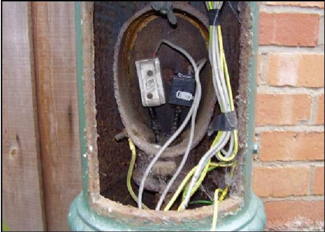
Exposed wiring emergency, see note 1: Target Response Time Cat E.
