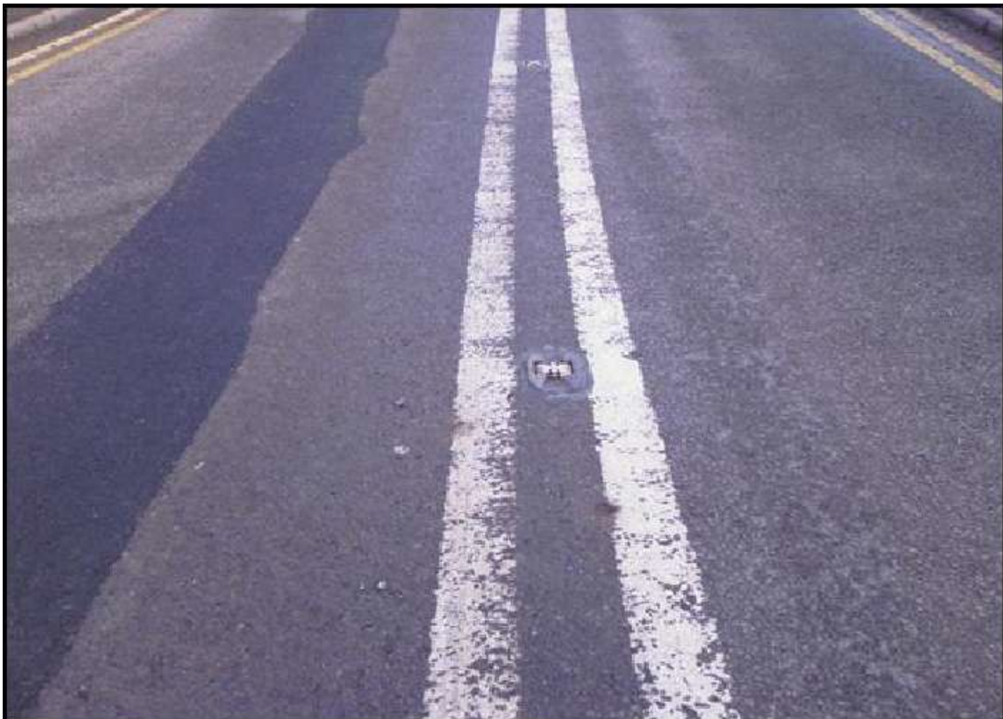
Worn double line system on a Secondary Distributor, see note 2.
