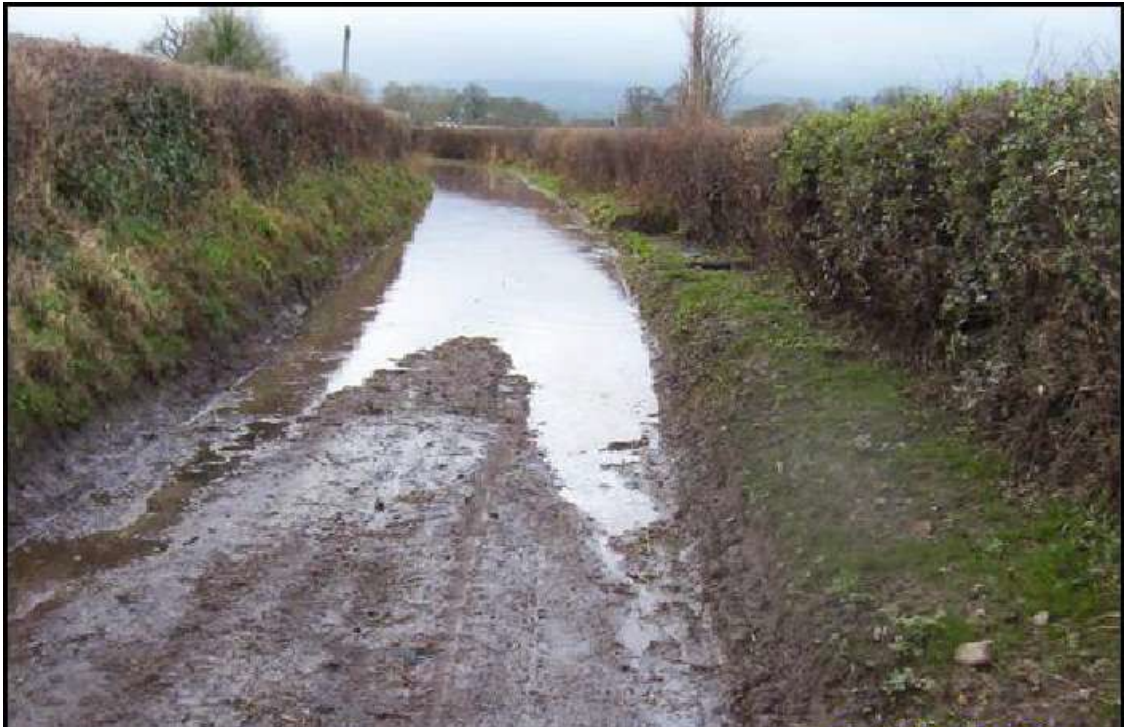
Flooded Local road, see note 2.
