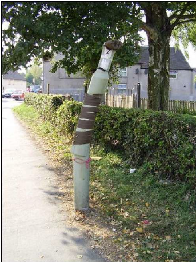
Damaged column, see note 1: Cat E.
