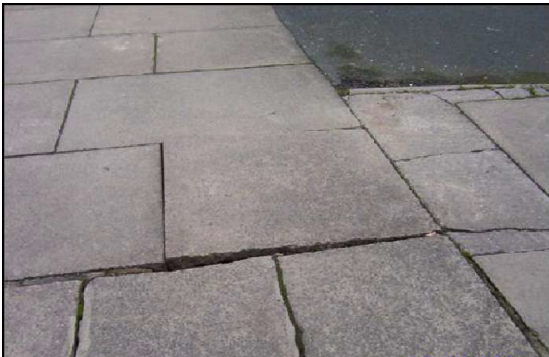
Displaced slab, Secondary Walking Route, Type 2: Target Response Time Cat 3.
