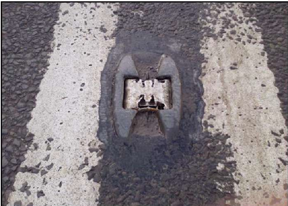
Worn catseye, double line system, see note 2.
