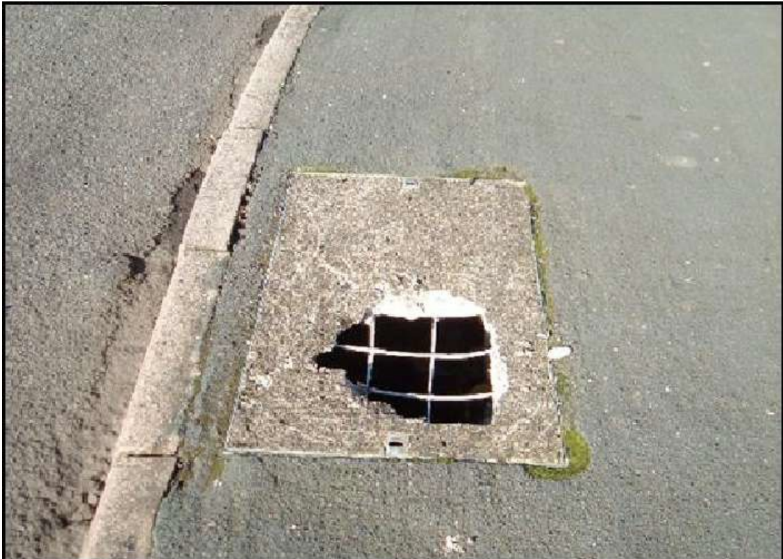
Broken BT cover Local Access: Target Response Time Cat E.
