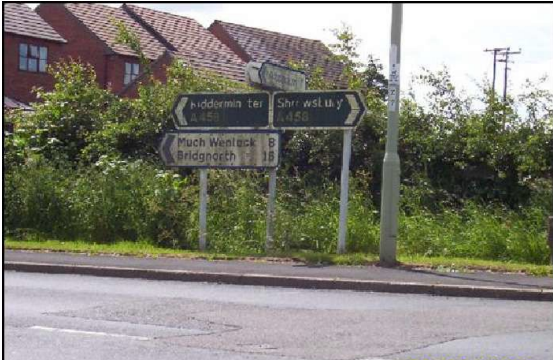
Worn direction signs on Strategic Route, see note 2.
