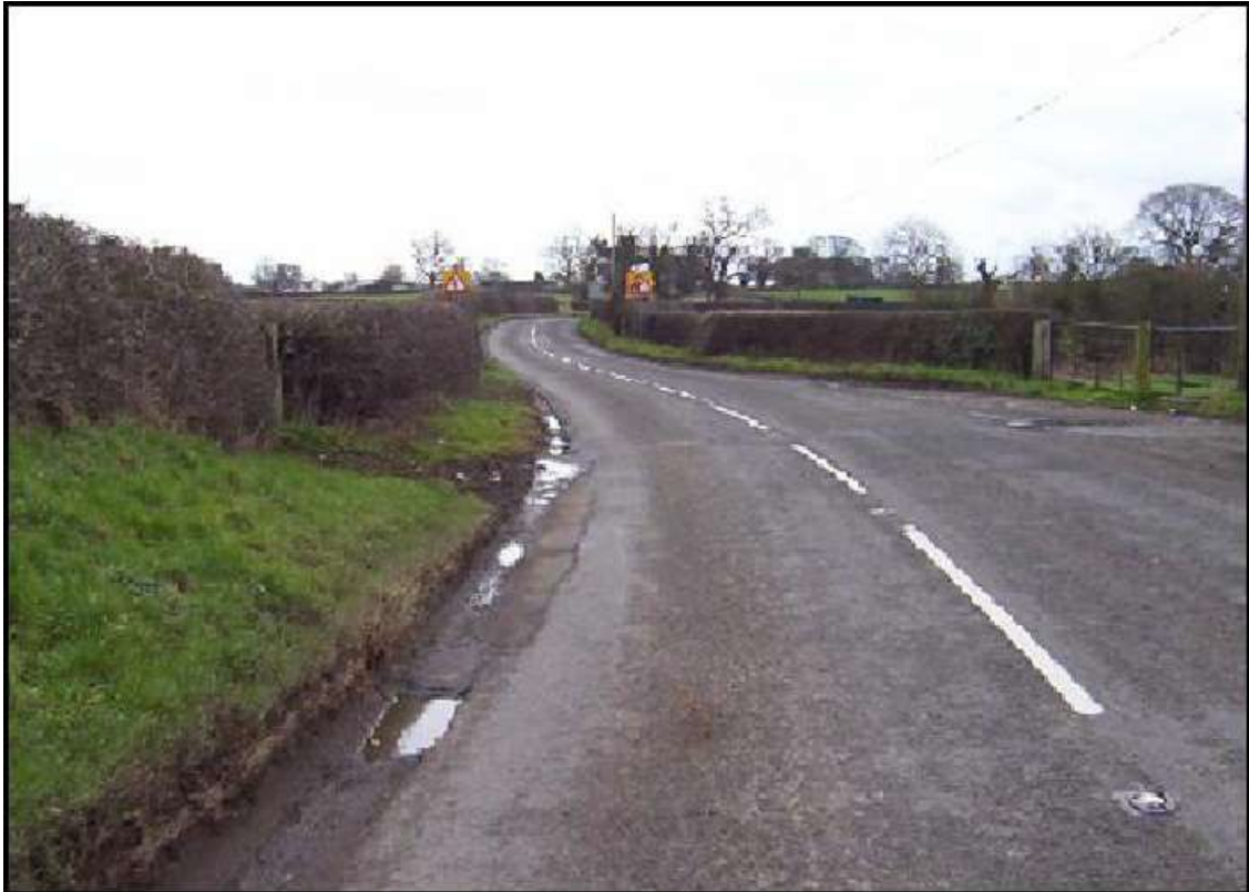
Edge deterioration Secondary Distributor, Type 3 defect: Target Response time Cat 2.
