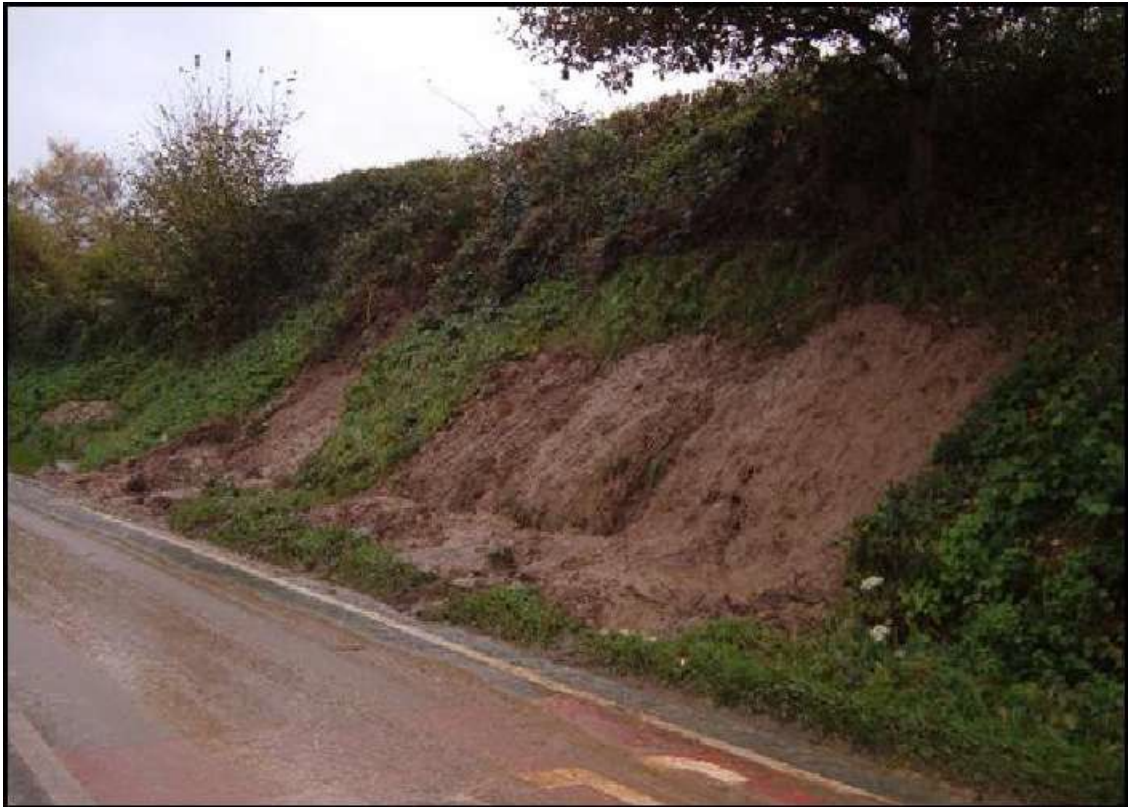
Landslide, storm damage see note 2.
