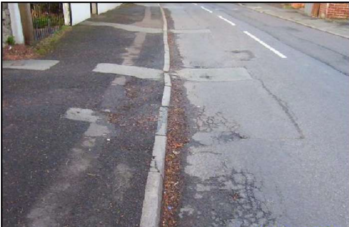
Footway surface and kerb problem, include in renewal programme.
