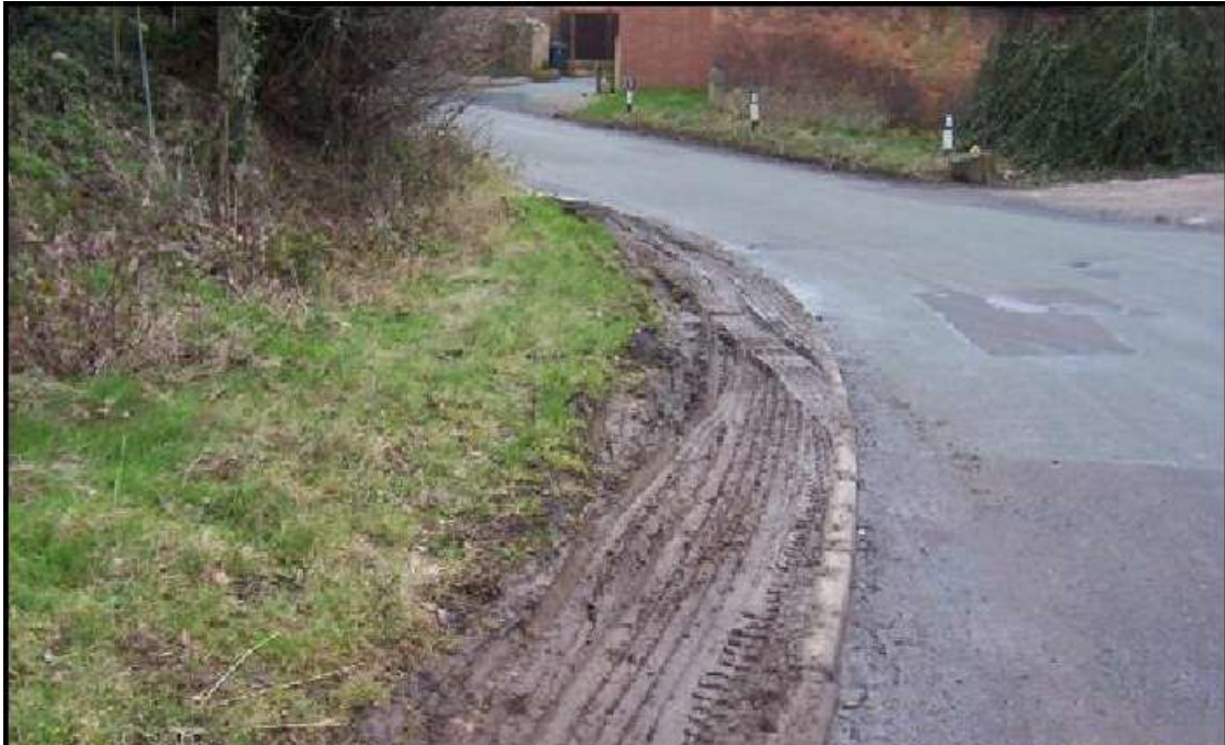
Footway damaged by over-running, include in renewal programme.
