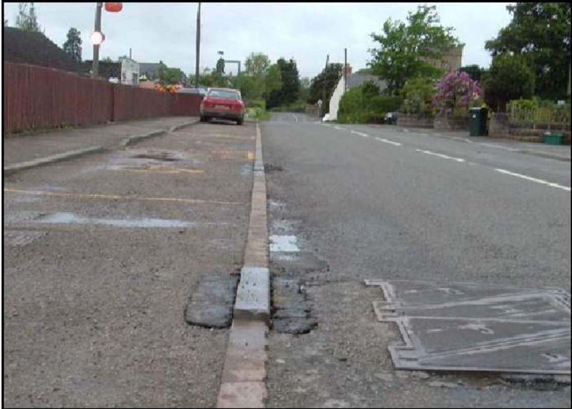
Damaged kerb, make safe with bituminous material and include in spot kerb replacement programme.
