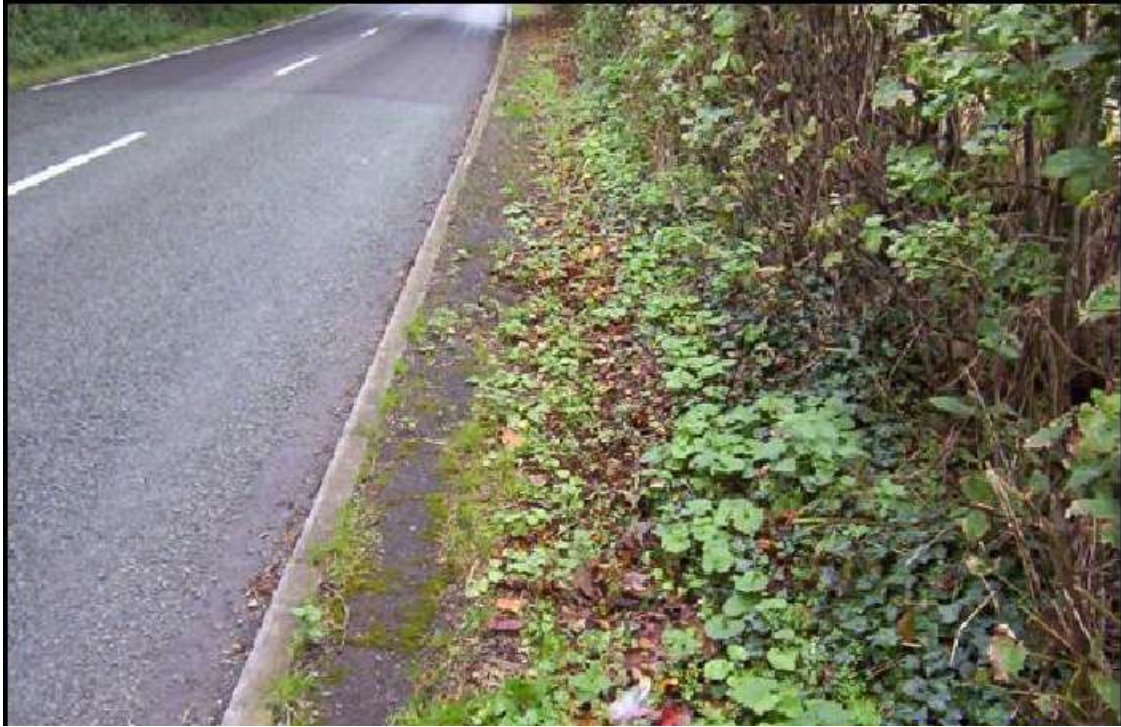
Little used rural footway overgrown by vegetation. Include in a siding programme when more than half of the footway overgrown.
